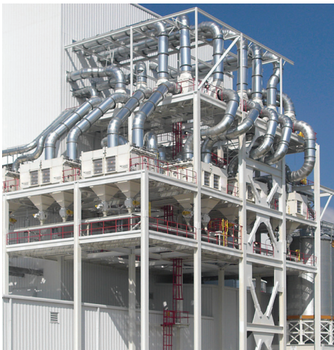
Multiple dust collectors in use at a grain processing operation.
